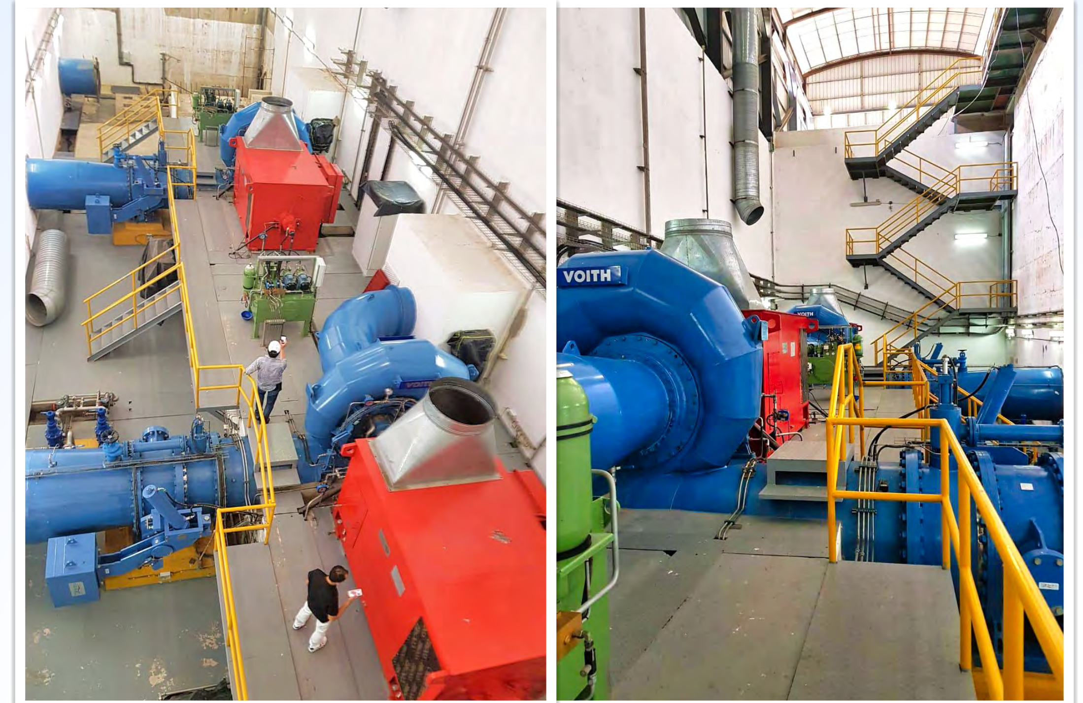
12MW Hydro Plant , 6MW planned extension Panama
